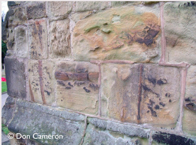
The Coal Measures Sandstone walling of the south aisle of the Church of St. Helen, Trowell is highly ferruginous, being seen to contain clasts as well as discrete bands of ironstone.
